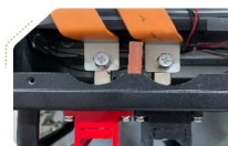
Battery internal and external connection
